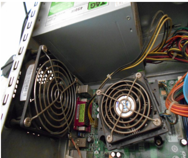
Fig.4: Fans used to cool internal air of the enclosed CPU
