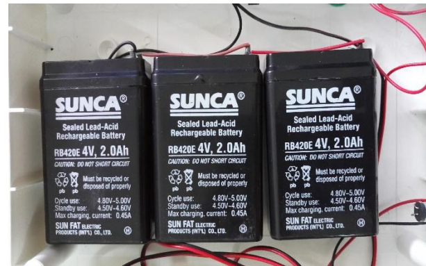
Fig 6: 4V lead Acid Rechargeable Battery Connected in Series.
